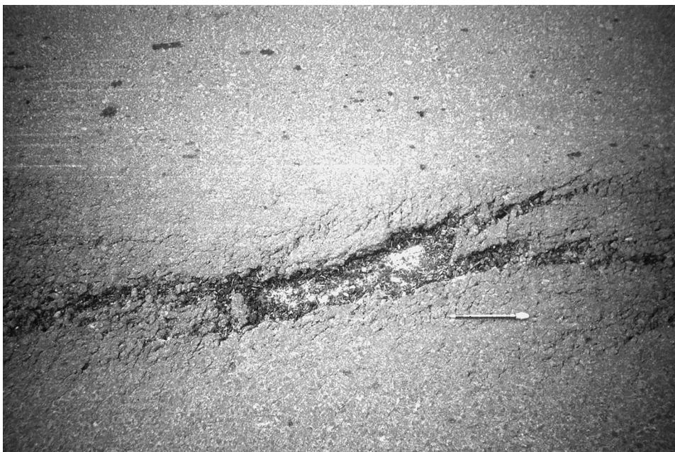
Fig. 5. A close-up of one of the pull-apart 'basins' that developed along the sinistral, strike-slip dislocation in the asphalt. The pencil measures ca. 15 cm.
